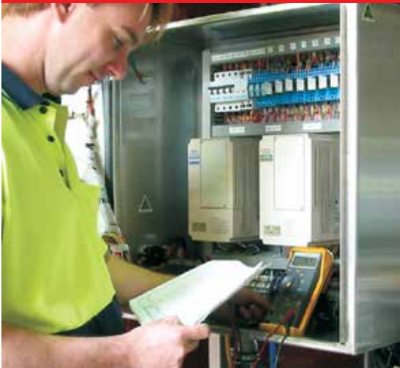
ELECTRICAL PROGRAMMING & TESTING
